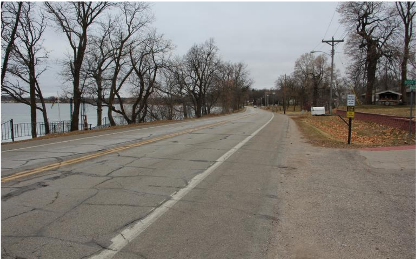
The pavement on West Lake Drive is in poor condition, one of the reasons city and county engineers would prefer to get it replaced.
